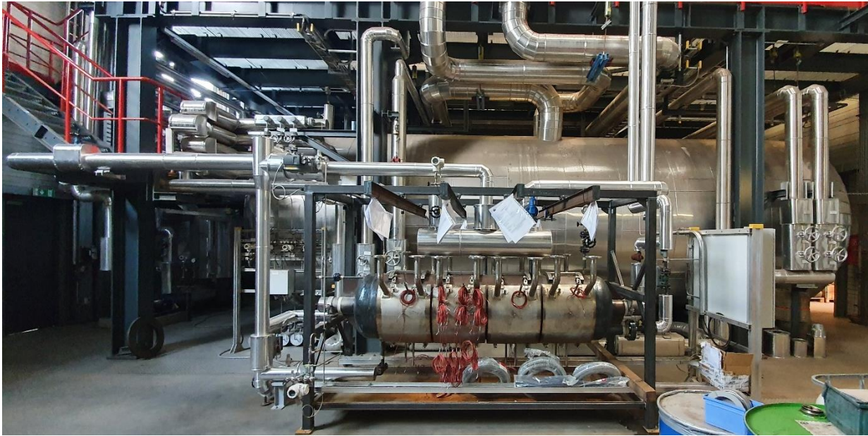
Figure 4.17: Module assembling onto the Lab scale Ruths steam storage device, in the background a 80 m³ Ruths steam storage device
