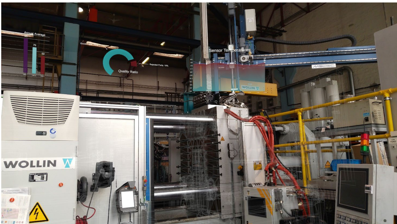
Figure 44: Dedicated parameters of the die casting machine can be controlled hands-free via Augmented Reality by using a dedicated communication protocol between Unity and the B&R process control system.
