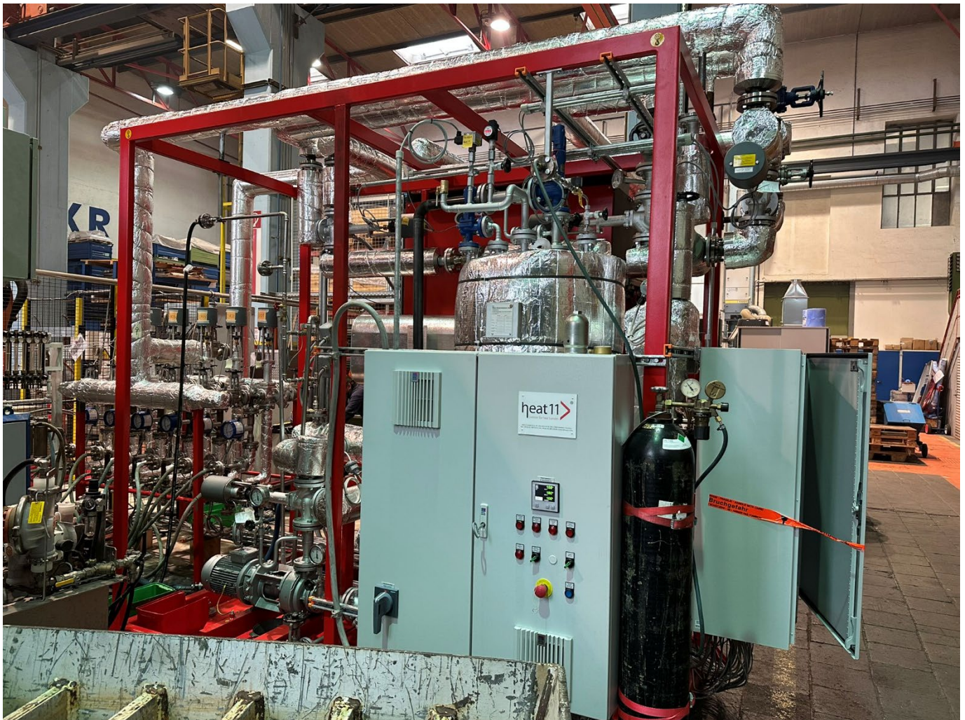
Figure 32: Central heating and cooling system of the Green Foundry 4.0 demo factory at LKR Ranshofen as delivered by heat11 according to the design and specifications of AIT.
