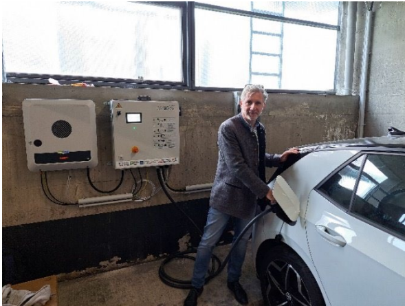
Figure 82: Charging Point EVN Garage
