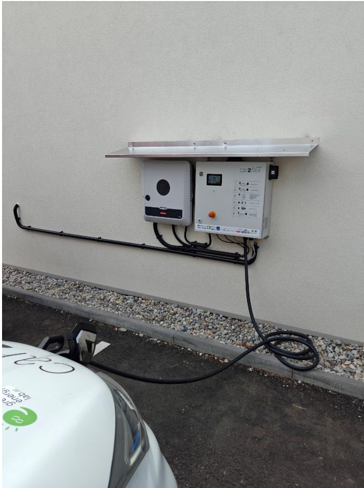
Figure 75 Charging station at Korneuburg
