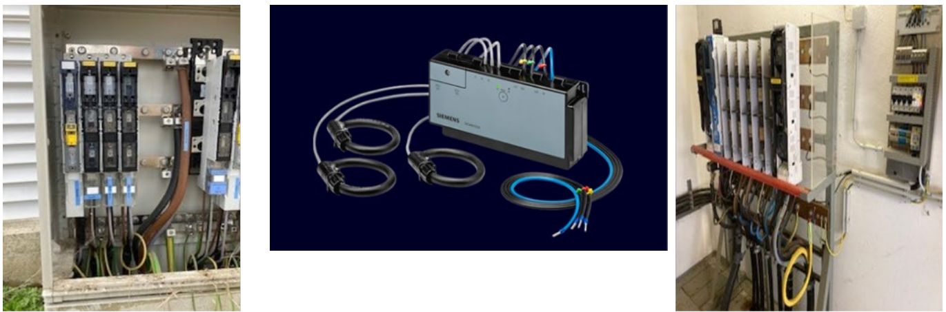
Figure 87 Grid Senors and Transformator-Installations
