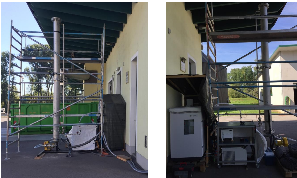
Figure 5 Pilot plant for siloxane removal on the wastewater treatment plant in Tulln
