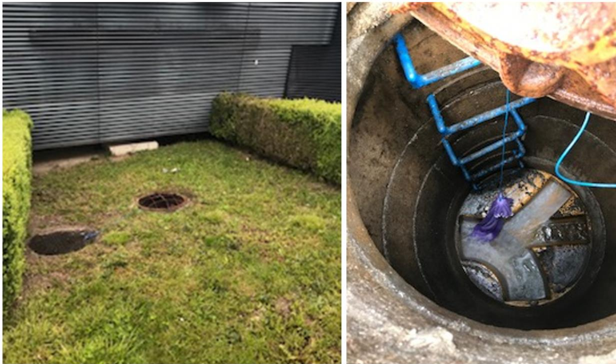
Figure 23: Shafts of the waste water system and waste water temperature measurement at Salesianer Miettex
