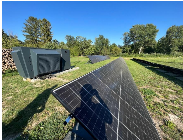
Figure 01: Line-up of the energy cell Johann at the farm yard in Pischelsdorf (Lower Austria)
